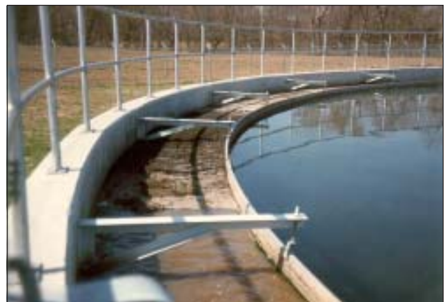
The race skirt traps floating scum within the race and prevents flow directly to the effluent weir.
